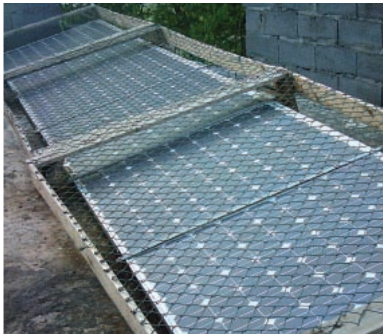
Fig. 4. Painéis fotovoltaicos, As Hortas, Fogo (Foto Capuano, 2008)
